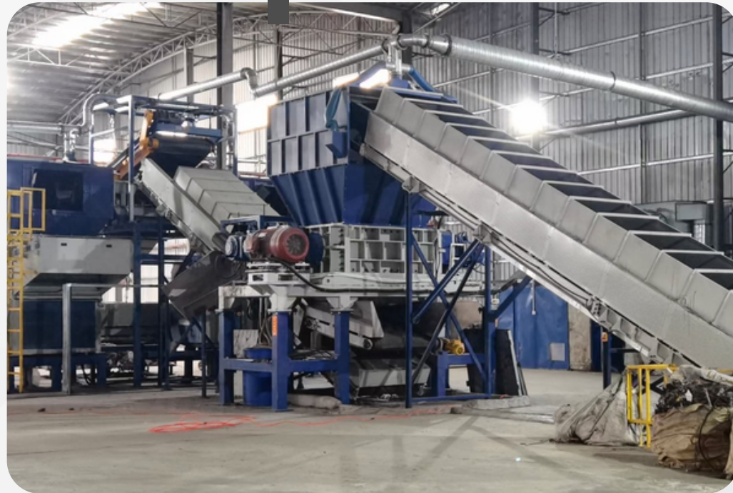
PRE-PROCESSING / SEGREGATION OF FUEL
