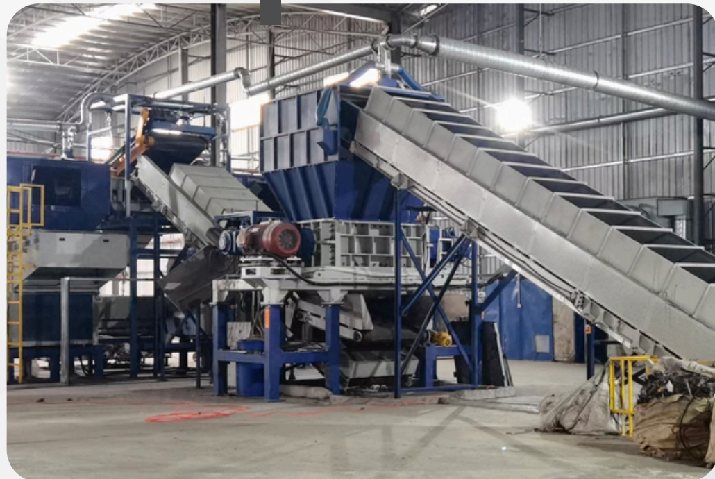
PRE-PROCESSING / SEGREGATION OF FUEL
